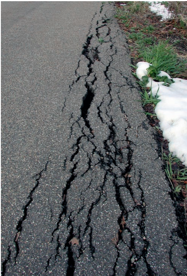
Figure 8.37 Extension fracture population along the edge of a paved road. Each of the fractures has grown from microfractures and they have reached a variety of sizes. The pavement is now more or less saturated with fractures, implying that additional strain will be accommodated by coalescence of existing fractures rather than by the nucleation of new ones.
