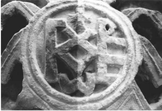
FIGURE 8.15 Encrustation cleaning from stone façade using the 3rd harmonic of a Q-switched Nd:YAG laser at 0.4 and 0.5 J/cm 2 . (Taken from Marakis, 2000.)
