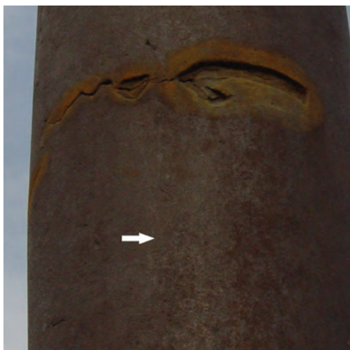
Figure 4. Localized corrosion below the dent on the pillar due to rust initially formed at the periphery of the dent and cracks. Arrow indicate areas where pits have formed below the dent.
