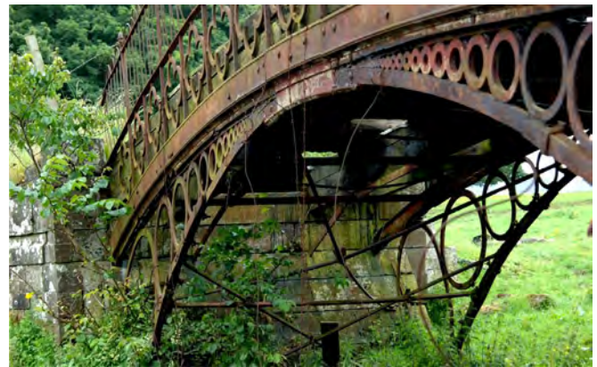
Figure 7. Close up view of damaged Linlathen East Bridge.
