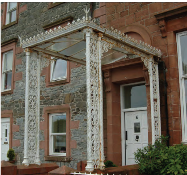
Figure 1. 19th Century hotel entrance canopy in poor condition. Isle of Bute, Scotland.
