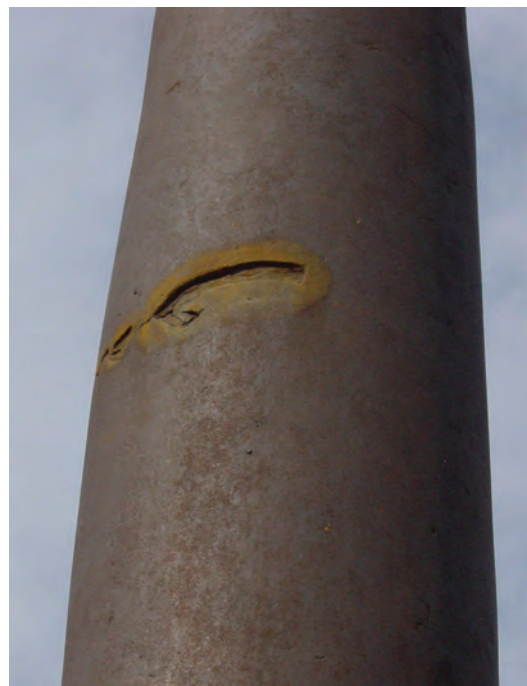
Figure 5. No pitting corrosion has formed above the dent on the pillar.
