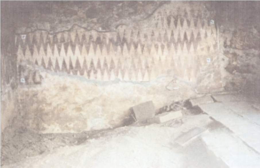
Figure 1. A view of red zigzag painted Plasters in a room of Alanya Castle Palace (ALP2).
