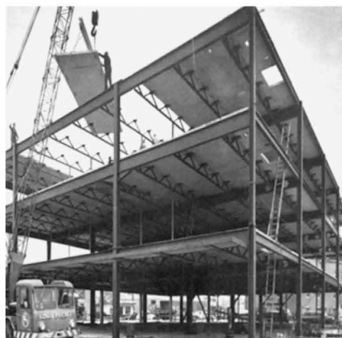
Fig. 12: Primary structure of (solid) rolled sections, secondary structure of (open) lattice beams
