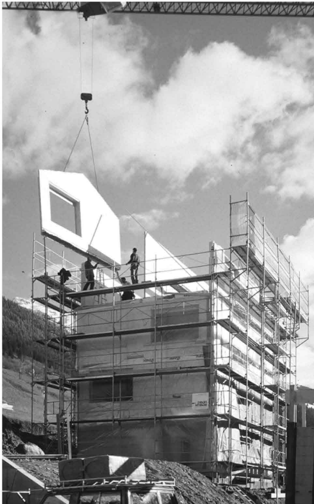
Figs 1 and 2: Solid timber panel construction, completed with shingle cladding (top); erecting the panels (bottom) Bearth & Deplazes: private house (Bearth-Candinas, Sumvitg (CH), 1998
