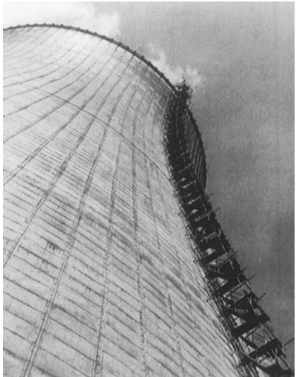
FIGURE 5.6 “Tubelox” tube and coupler scaffolding with integral step units for access to 330-ft-high curved stack. The step units are available with guardrail and midrail panels, plus the opportunity of positioning landing or rest platforms at any desired level.
