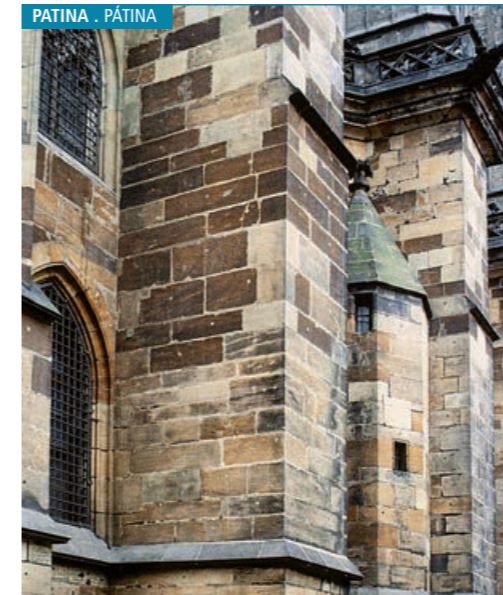
The sandstone elements of these buttresses show a variety of colours. Creamy to orange colours correspond to stones more recently set into the masonry. Brown colours are due to the development of an iron-rich patina, as a result of a longer exposure in the open air.
