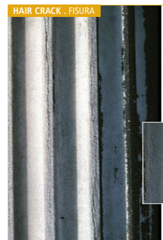
HAIR CRACK . FISURA
