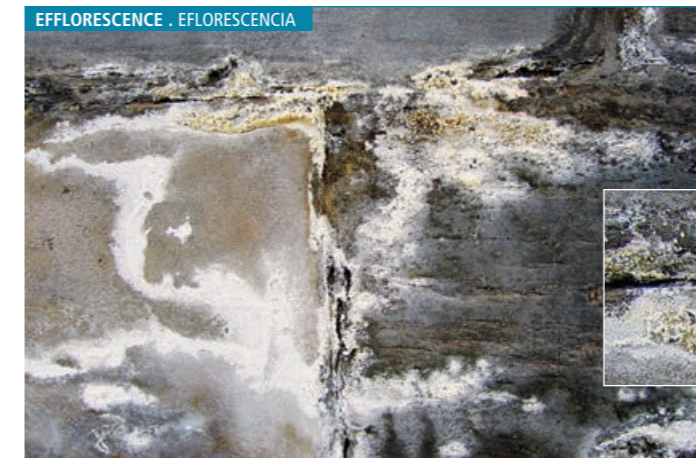
Formation of salts forming efflorescence on the surface of sandstone masonry, focused at joints between masonry blocks.
