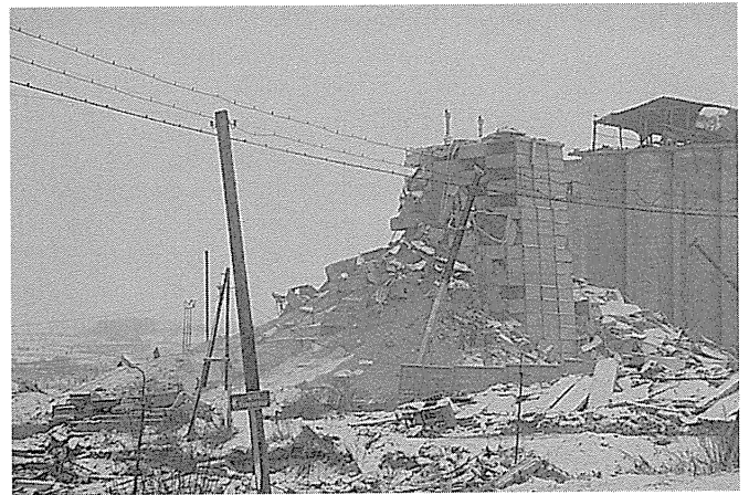
Fig. 1.2-7 Five-story building in Spitak, Armenia, destroyed during the December 7, 1988, earthquake. The building was made from precast concrete frames that were inadequately connected. The failure of such buildings contributed greatly to the loss of 25,000 lives. (Courtesy of the US Geological Survey.)
